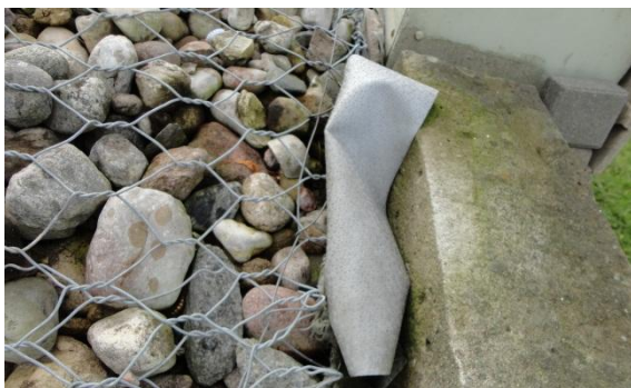
Figure 8. Waterproof membrane with no connection to structural element (Source: photo by the authors, 2012)
